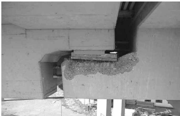
Fig. 2.11—Damage at Fourth Avenue on-ramp in 2001 Nisqually earthquake. (Courtesy of Washington Department of Transportation.)
