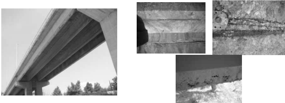
Figure A5 : Typical deck of the approach viaducts and visible corroded reinforcement at the bottom flange of the deck beams, concrete corrosion at the area adjacent to gutters and , porous at the bottom flange of the prefabricated beam
