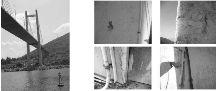
Figure A4 : Pylon M5 – General view and concrete damages e.g. delamination with corroded reinforcement at the column, cracks at previous concrete repairs, delamination at the area of the manhole of the pylon, visible corroded reinforcement at the base of the pylon
