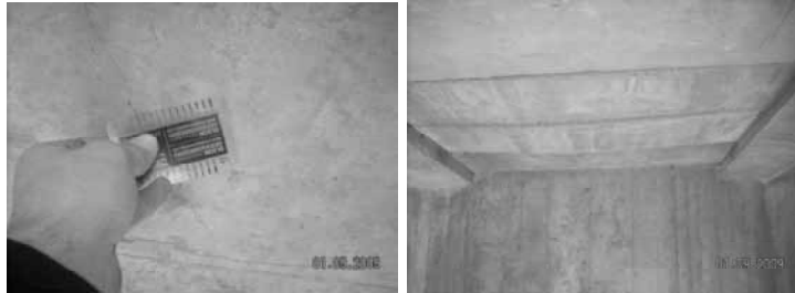
Figure A8: Very small crack and visible deflection at the pre-slabs
