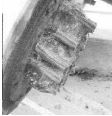
Figure 9: Bottom anchorage head. The integrity and the good status of the cement grouting are visible.
