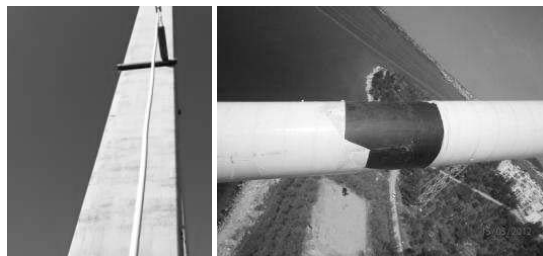
Figure A10 : Waving of the cable pipe (not the strands) due probably to loose hanging during construction, minor damage of the protection tape; the 44% of the stays presented such small damages of length up to 50cm
