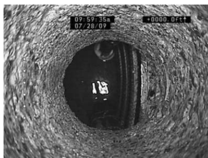
Figure 8: Defect seen from a core hole
