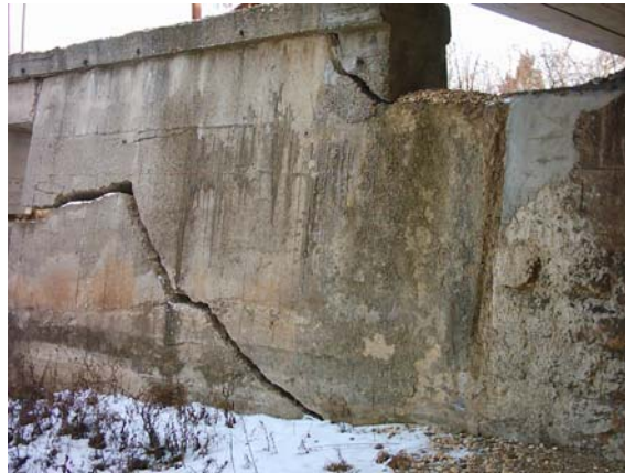
Fig. 17. Large crack in the lateral retaining wall of the bridge near Makotzevo
