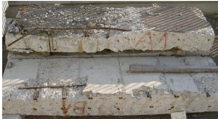
Fig. 20: View of the slab specimen cut from the bridge deck
