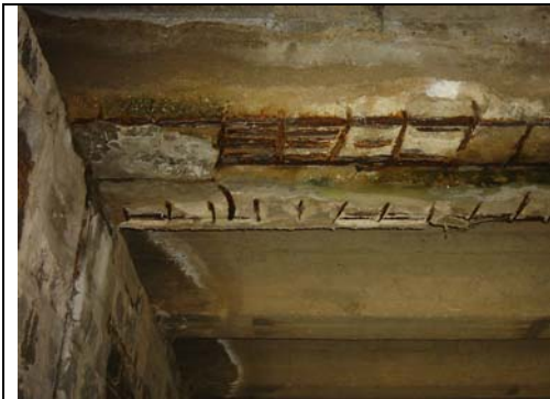
Fig.13: Railway bridge near Mircovo showing heavy rusting of the reinforcement due to cyclic wetting and freeze – thaw.
