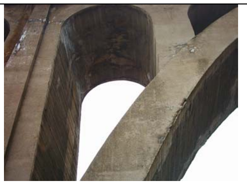
Fig. 16. Bridge near Klisura with evidence of steel rusting on the lower surfaces
