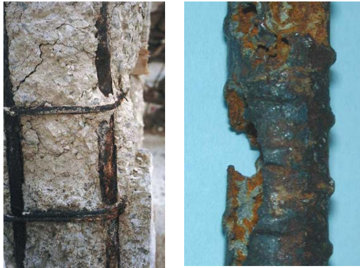
Fig. 4. Effects of the carbonization and pitting corrosion on the reinforcement
