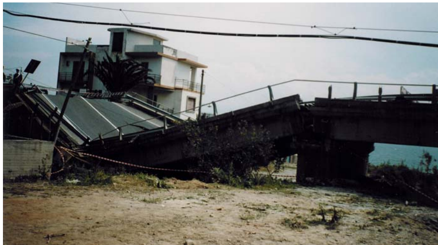
Fig. 5: Collapse of the Saint Stephan bridge due to pitting corrosion of the main bars
