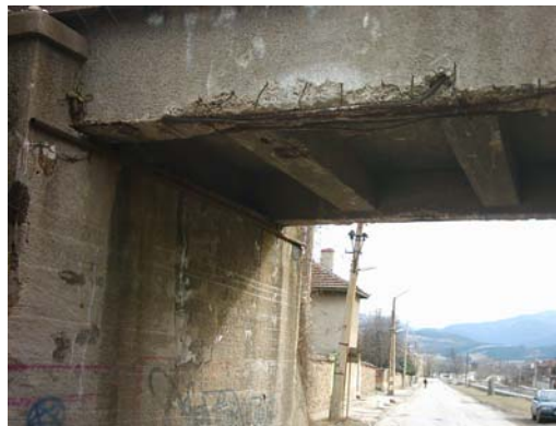
Fig. 12: Railway bridge in Chelopech showing reinforcement corrosion due to weather exposure after a vehicle impact
