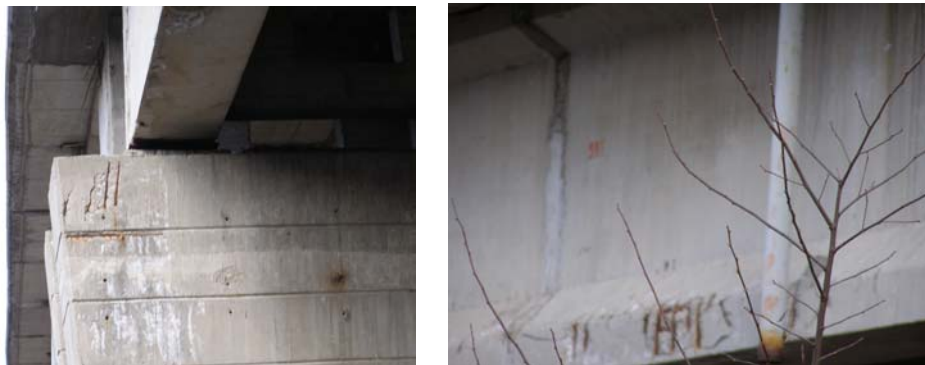
Fig. 11: Cover detachments showing the start of corrosion in two viaducts in “Trakia-Highway”
