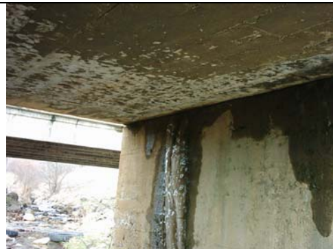
Fig. 14: Water flowing through the dilatation joint at the bridge abutment between the Pirdop and Anton station stops.
