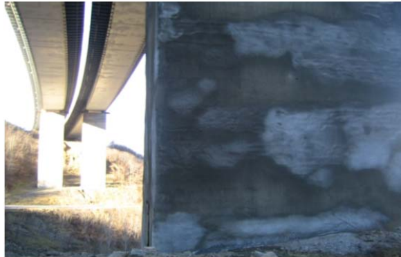
Fig. 10: Sprayed concrete repair of one pier in the steel structure viaduct near the central 162 m span
